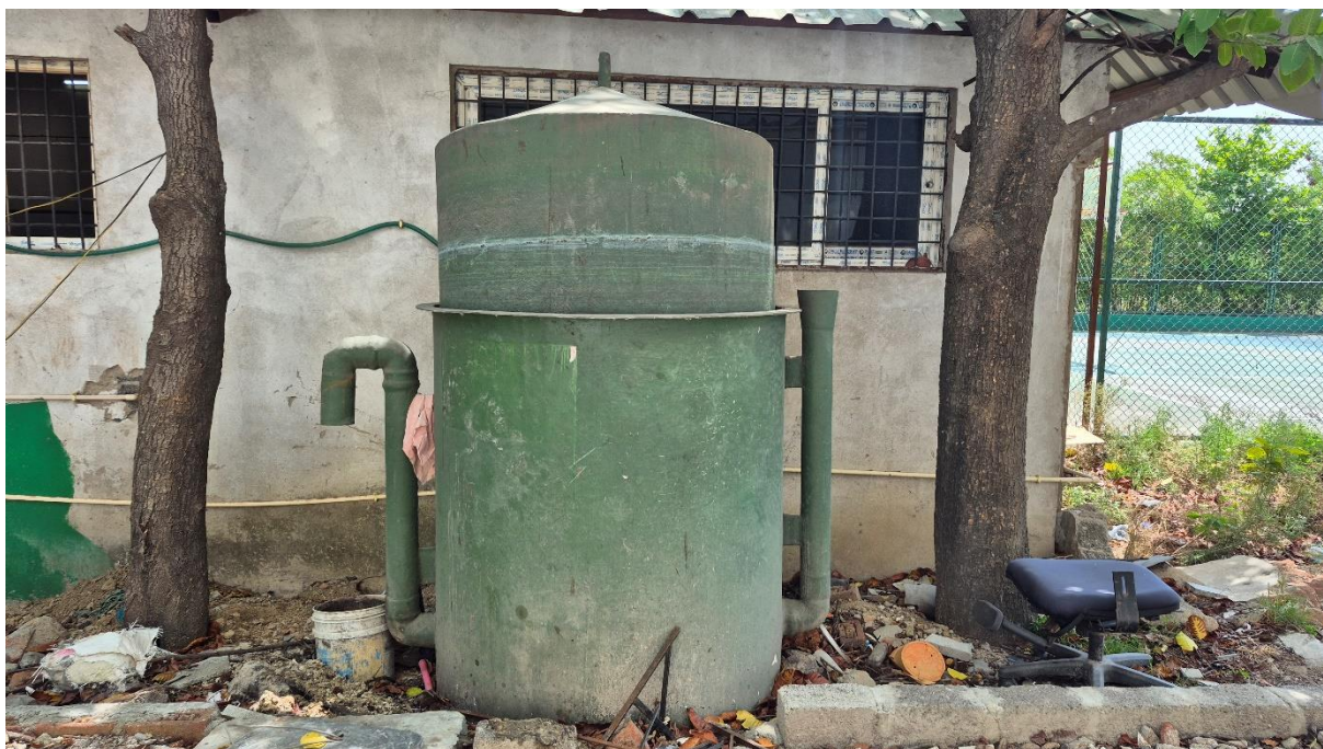
Sewage Treatment Plant at IARE
