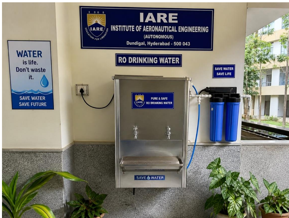
RO Water Facility at IARE
